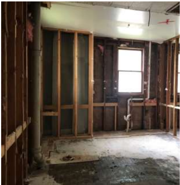
A view of the main level bathroom (left) and corner of the office (right) after initial demolition.
