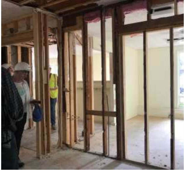
The wall between the coat racks and the sunroom is being removed to create the new lobby.
