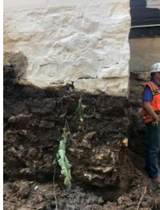
Excavation along the furnace room wall revealed that the wall did not reach the basement floor level or have a footing. This area will need to be underpinned with concrete to provide adequate support for the existing wall and to create an adequate base for the new addition.
